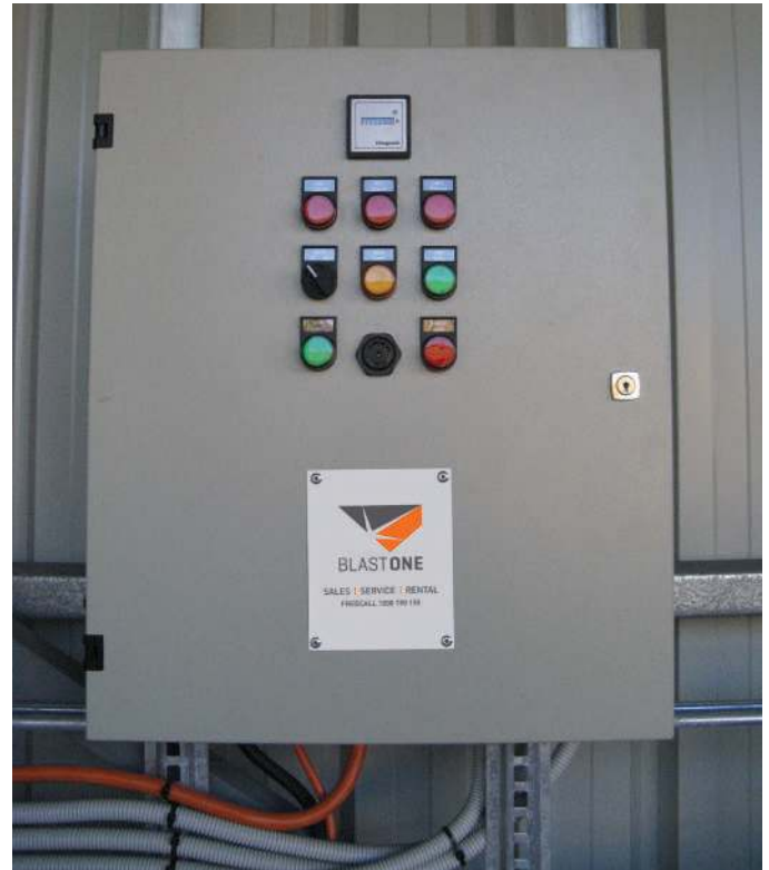
TRIPLE EXTRACTION FAN SYSTEM CONTROL BOARD
