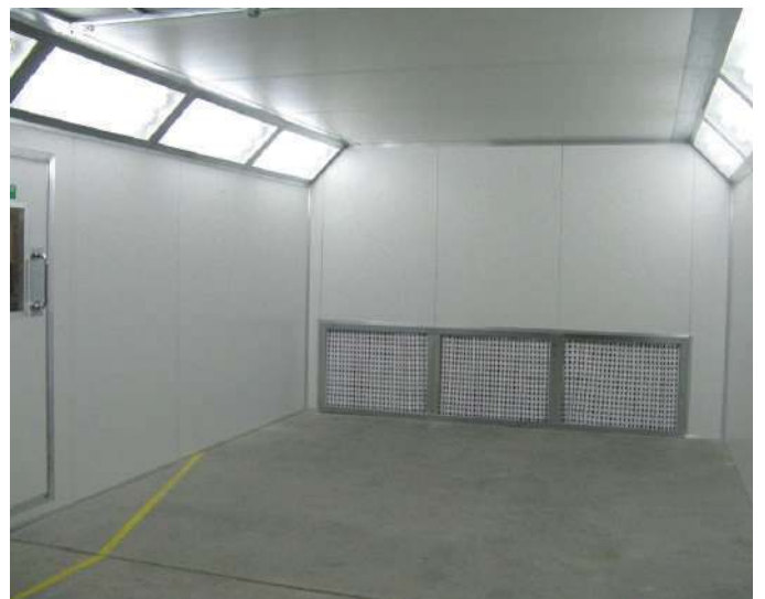
INSIDE DETAIL OF A SEMI DOWN DRAFT SPRAY BOOTH/CURING OVEN
