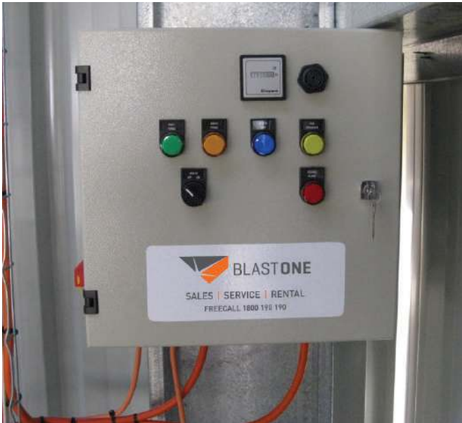
SINGLE EXTRACTION FAN SYSTEM CONTROL BOARD
