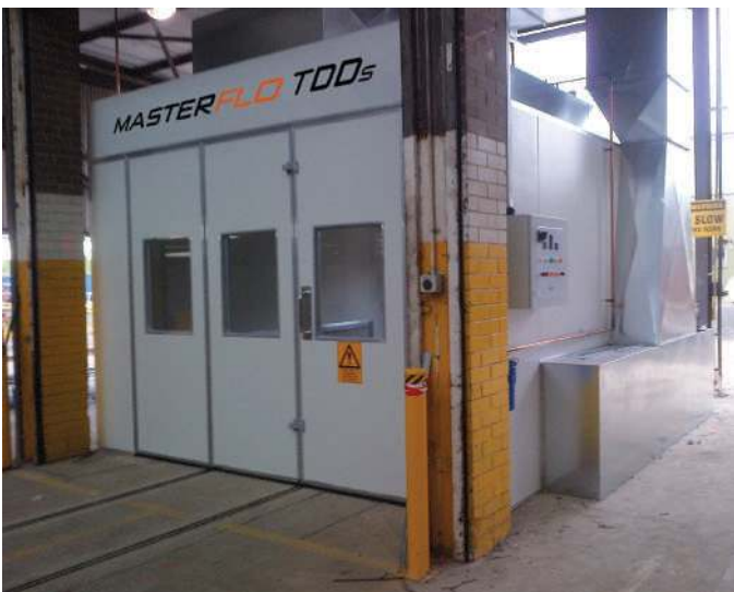
SIDE DOWN DRAFT SPRAY BOOTH/CURING OVEN
